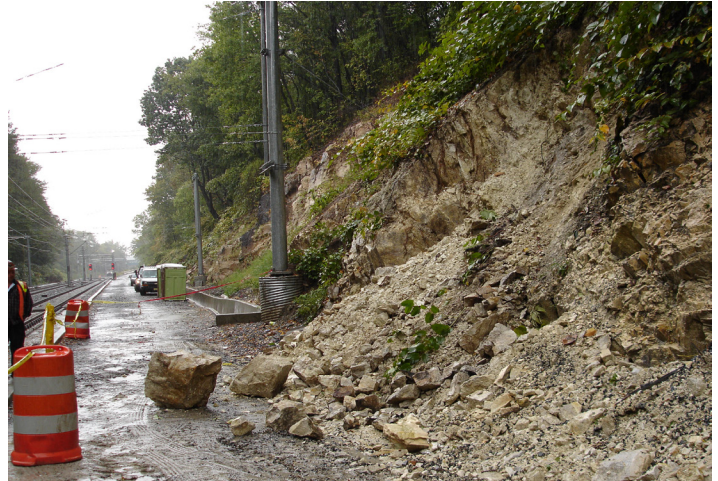
Figure 1. Unstable rock conditions leading to localized slope raveling near the West Portal.
