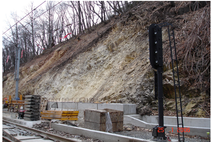
Figure 2. Construction of concrete block retaining wall near West Portal to stabilize raveling rock.
