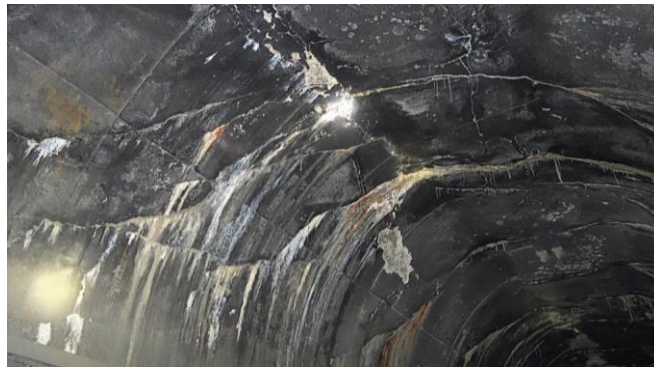
Figure 6: Typical damages in the tunnel's back
