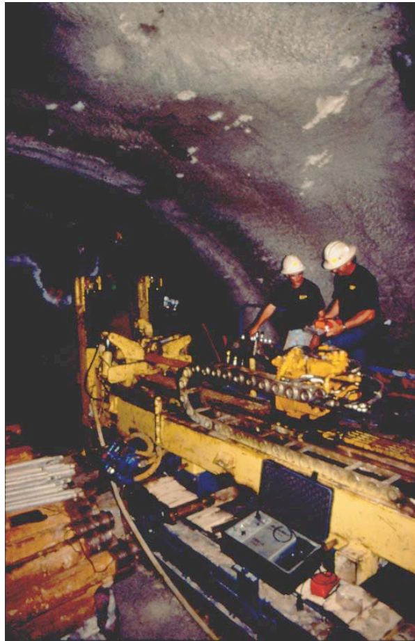
Figure 4 - Section E4b – Horizontal Directional Drilling (HDD) from within Drilling Chamber (Courtesy Paul Madsen, Kiewit Construction)
