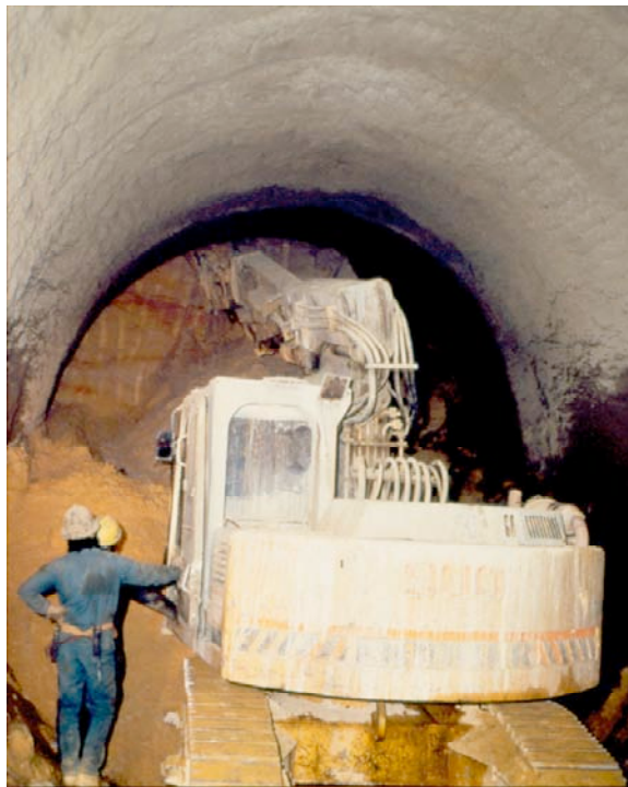
Figure 3 - Section E4b – NATM Tunneling under Rock Creek Cemetery (Courtesy Paul Madsen, Kiewit Construction)
