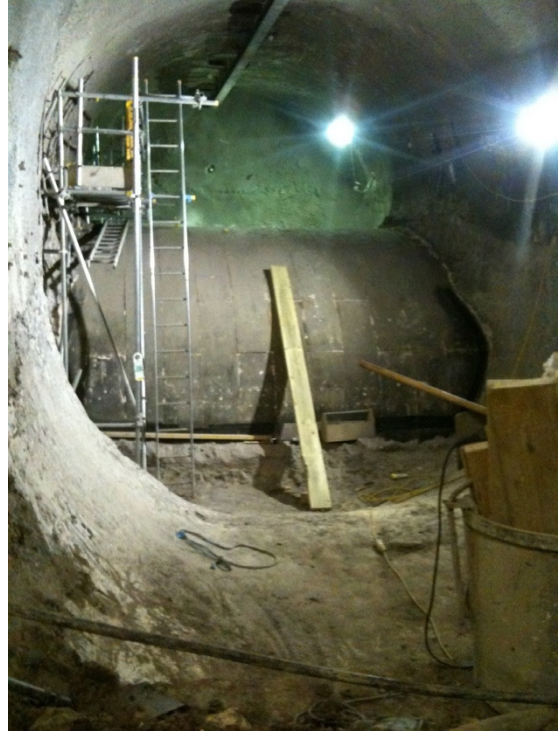
Figure 1. Excavation and Primary Lining completed for new Central Line over-bridge. (Courtesy of London Underground Ltd.)
