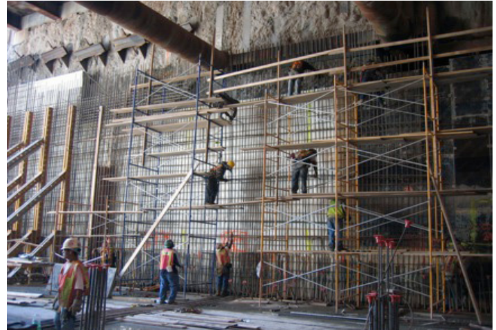
Figure 1. Waterproofing membrane placed on sidewalls and installation of reinforcing bars. (Courtesy of MTACC)
