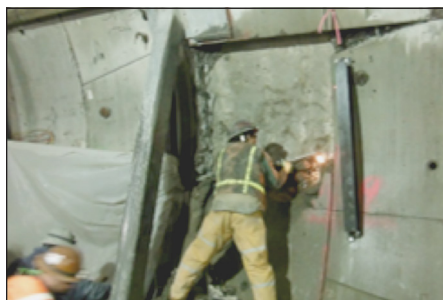
Exposed grout behind segment
