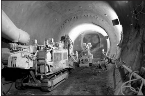
Figure 9. Grouted steel pipe arch installed underneath the Maidenlane Tunnel (Courtesy A. Reinhart)
