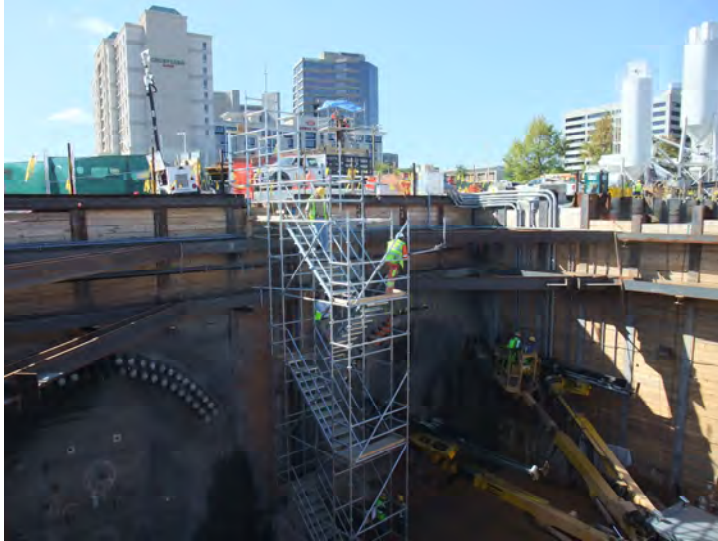
Figure 5. View NATM Tunnel East Portal in Relation to High-rise Buildings near the Alignment
