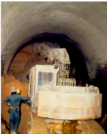
Figure 3. Section E4b – NATM Tunneling under Rock Creek Cemetery (Courtesy Paul Madsen, Kiewit Construction)
