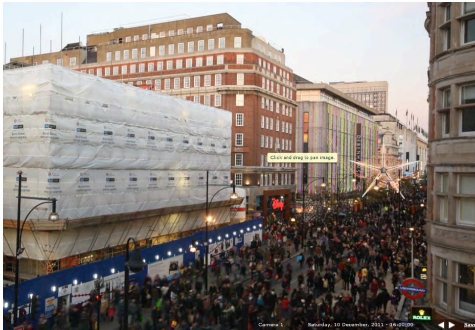
Figure 3 Busy Oxford Street with the building under demolition on the left hand for construction site area
