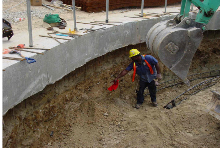
Figure 1. Excavation in soil underneath a cast-in-place concrete shaft collar to be followed by shotcrete for initial support reinforced by lattice girders (different angle).
