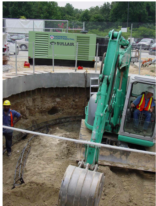
Figure 2. Excavation in soil underneath a cast-in-place concrete shaft collar to be followed by shotcrete for initial support reinforced by lattice girders.
