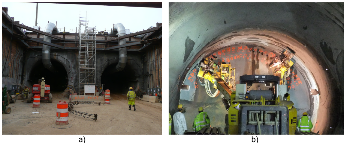
Figure 5. a) View into Inbound and Outbound Tunnels from East Portal, b) Installation of Pipe Arch Canopy in Outbound Tunnel
