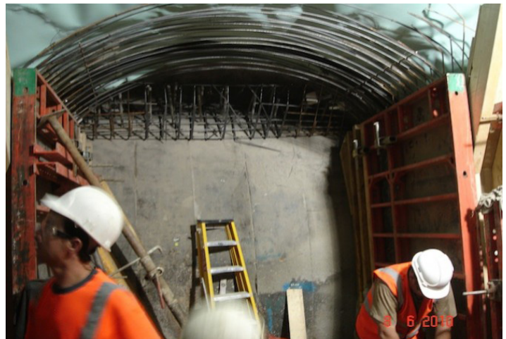
Figure 2. Preparations for installation of opening frame for connection into existing platform tunnel 3.
