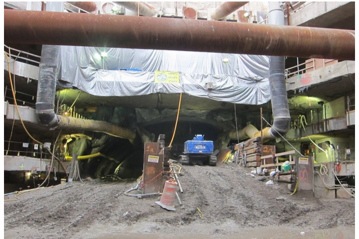
Figure 2. Drift 5 (center drift) excavation and support trailing behind Drift 1 (left drift) excavation and support.
