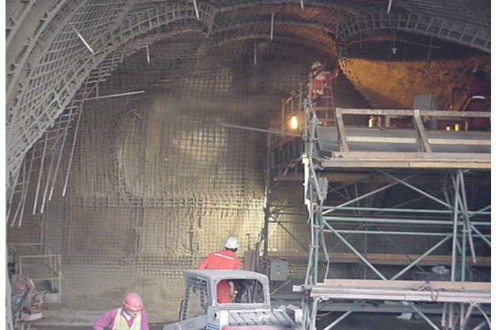
Figure 1. Installation of reinforced shotcrete final lining at the junction between the walkback and adjoining utility tunnel.
