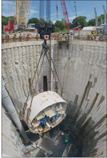
Figure 5. 375-ton TBM front shield lowered with the 600-ton crawler crane in the launch shaft
