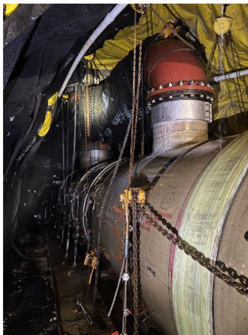
Figure 2. Hobas pipe connections to vent and drop shafts.
