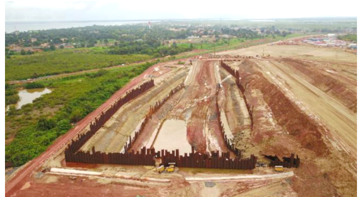
Figure 1. View from South of the excavation, showing the landslide on the right side (courtesy of GAC).
