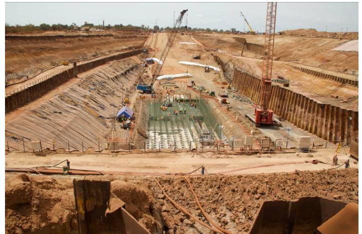
Figure 2. Car Dumper Excavation after the recovery of the excavation), during construction of the base slab.
