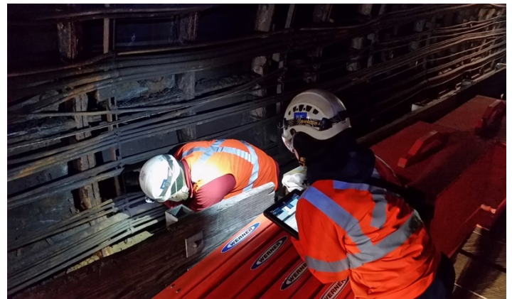
Figure 2. Measuring thickness of steel liner at locations of heavy corrosion.
