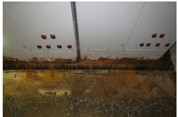
Figure 2. Leaking area in Bergenline Avenue Station.
