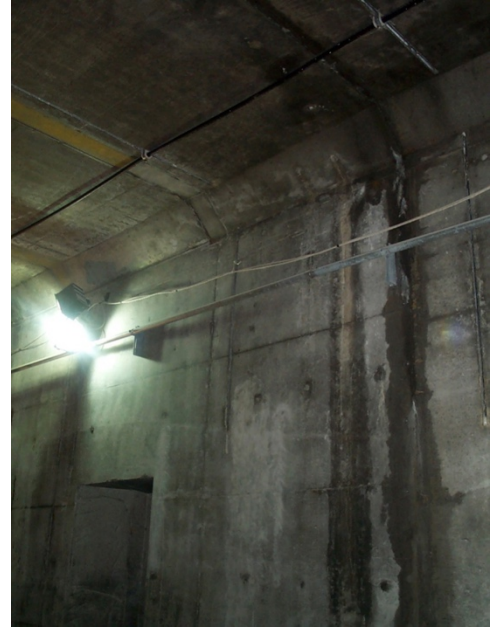
Figure 1. Leakages through a cracked concrete section.
