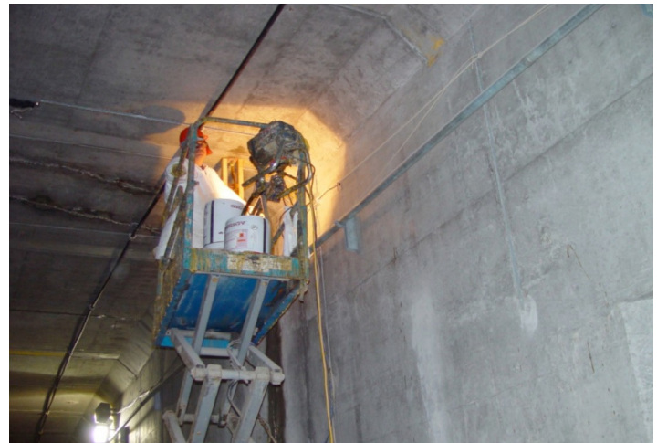
Figure 2. Grouting of the roof port (control and grouting pipe) into the roof compartment..
